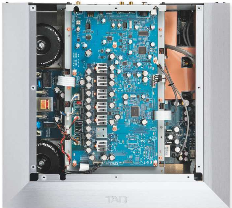
RIGHT: A single Burr-Brown PCM1794 DAC is visible on this top PCB which also carries a deal of PSU regulation for the various digital and analogue circuits. Note the unused, but ready-screened sections of the PCB
