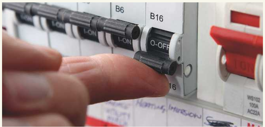
ABOVE: Switching an MCB (Micro Circuit Breaker) on a UK domestic electrical consumer unit. In the old days you had to cut appropriately rated fuse wire and refit it to your mains plugs
